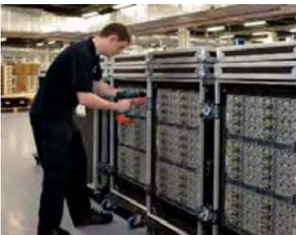
Data center and network deployment
