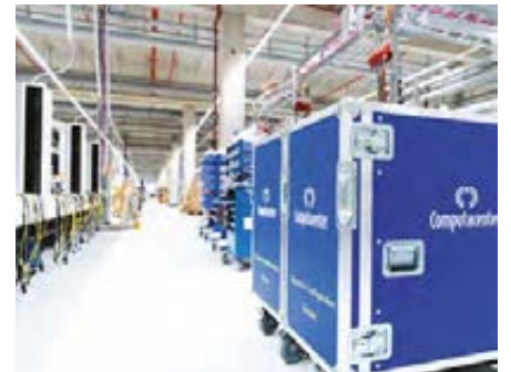
Data center and network deployment
