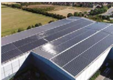
Solar panel installation – Hatfield, UK This is believed to be the largest rooftop installation in the UK in 2019.
